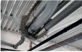
8-ways valves inside the rooms.
