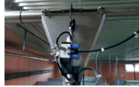
Actuated valve on feeding chains.
